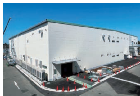
New wing of the Tsukuba Plant (Construction to be completed in July 2024)
